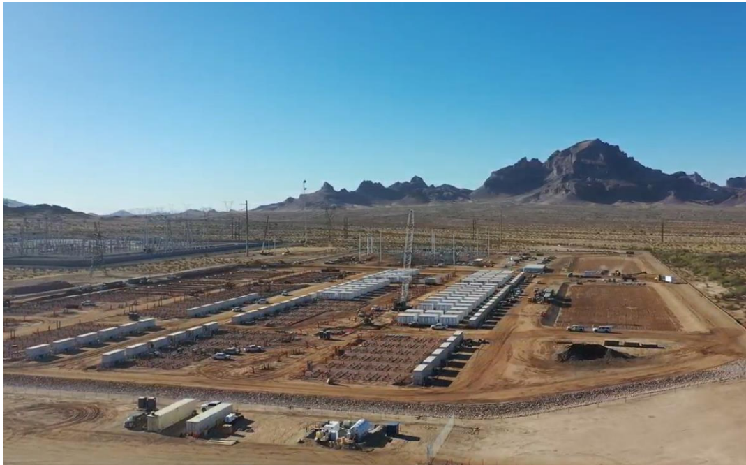
1,200 MWh Papago Storage Project located in Maricopa County, Arizona
